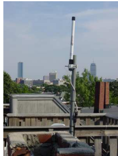
Figure 2: A typical Roofnet antenna installation. The cable leads to a node inside the building.
